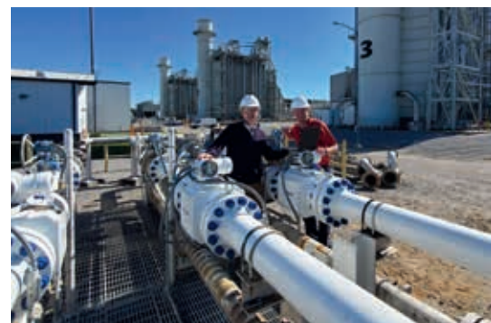
Custody transfer flow measurement for a natural gas fuel system
