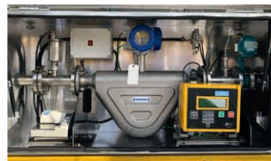
Custody transfer flow measurement of AdBlue® from road tankers
