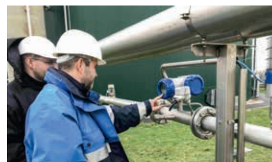
Instrument commissioning carried out by a KROHNE service technician
