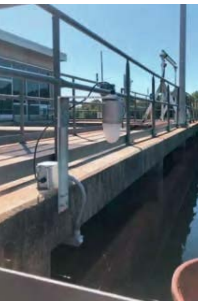
Radar level measurement of water basin
