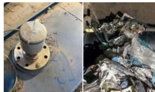
Level measurement of plastic waste in a waste treatment plant
