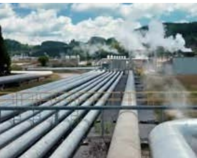
Geothermal steam measurement system
