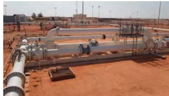
Custody transfer metering systems for produced water
