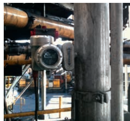
Tailings thickener underflow concentration measurement
