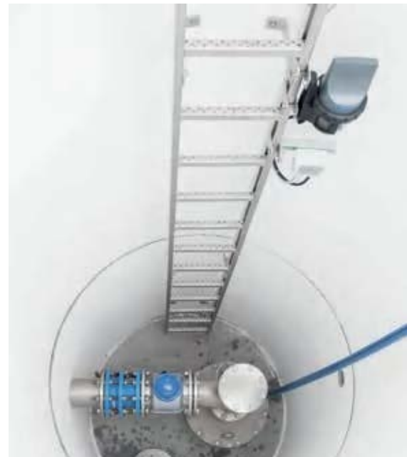
Battery-powered IP68 metering point with GSM/GPRS communication
